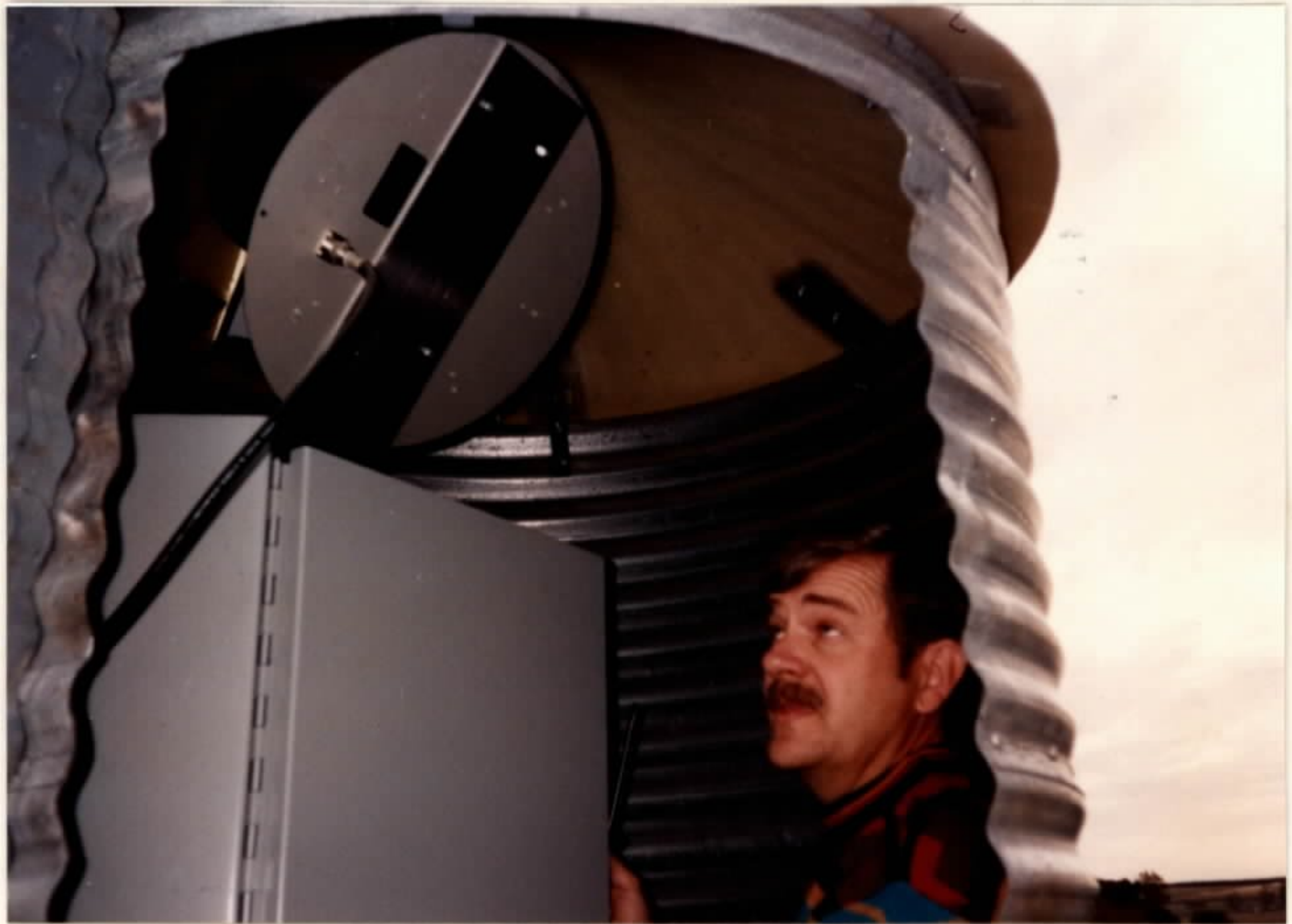
ALTERNATIVE INSTALLATION USED TO PROTECT THE ANTENNA AND THE SOLAR PANEL - LAKE LOWELL STATION -
