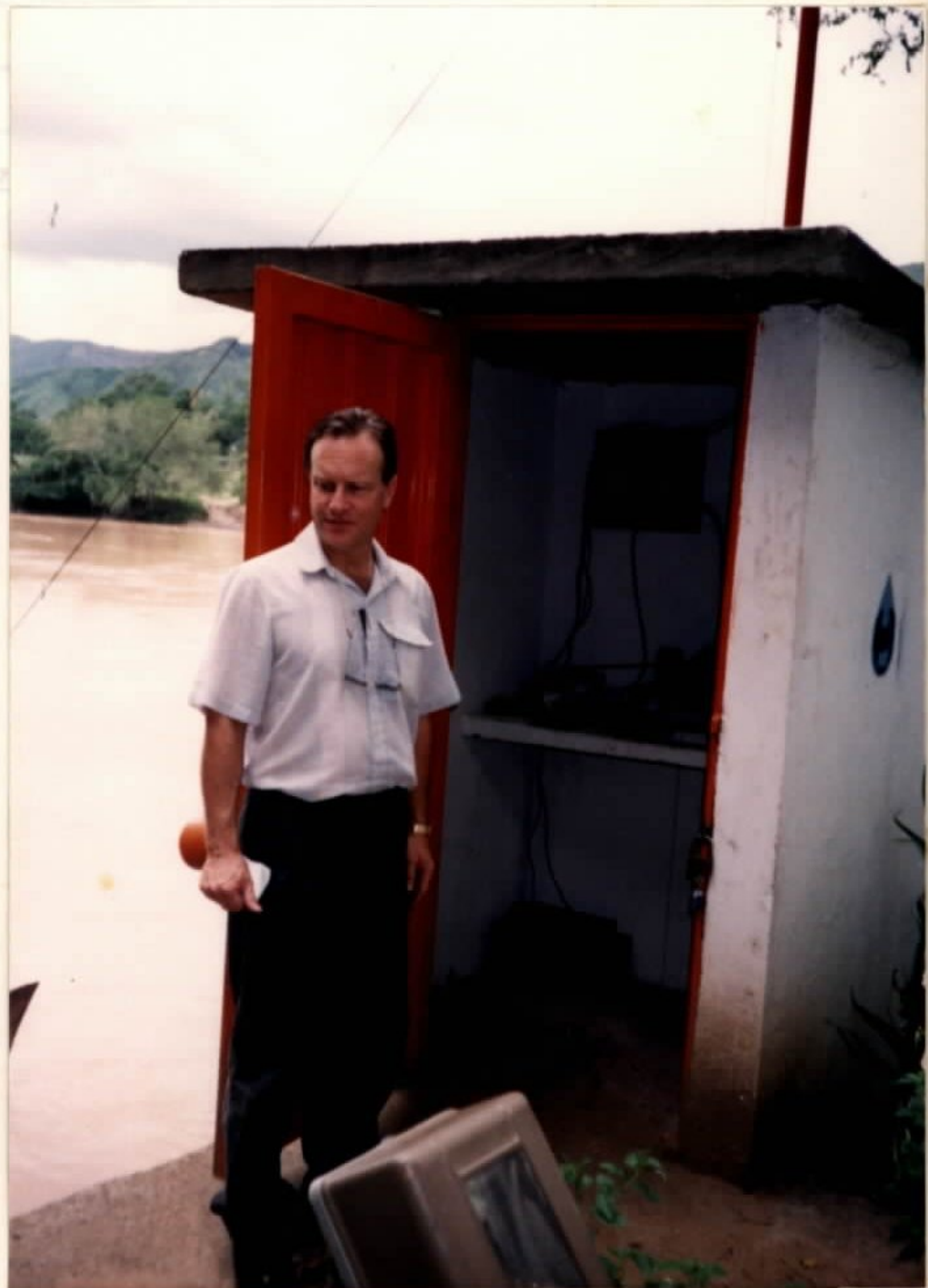
NARINO STATION BATTERY, SENSORS AND DCP
