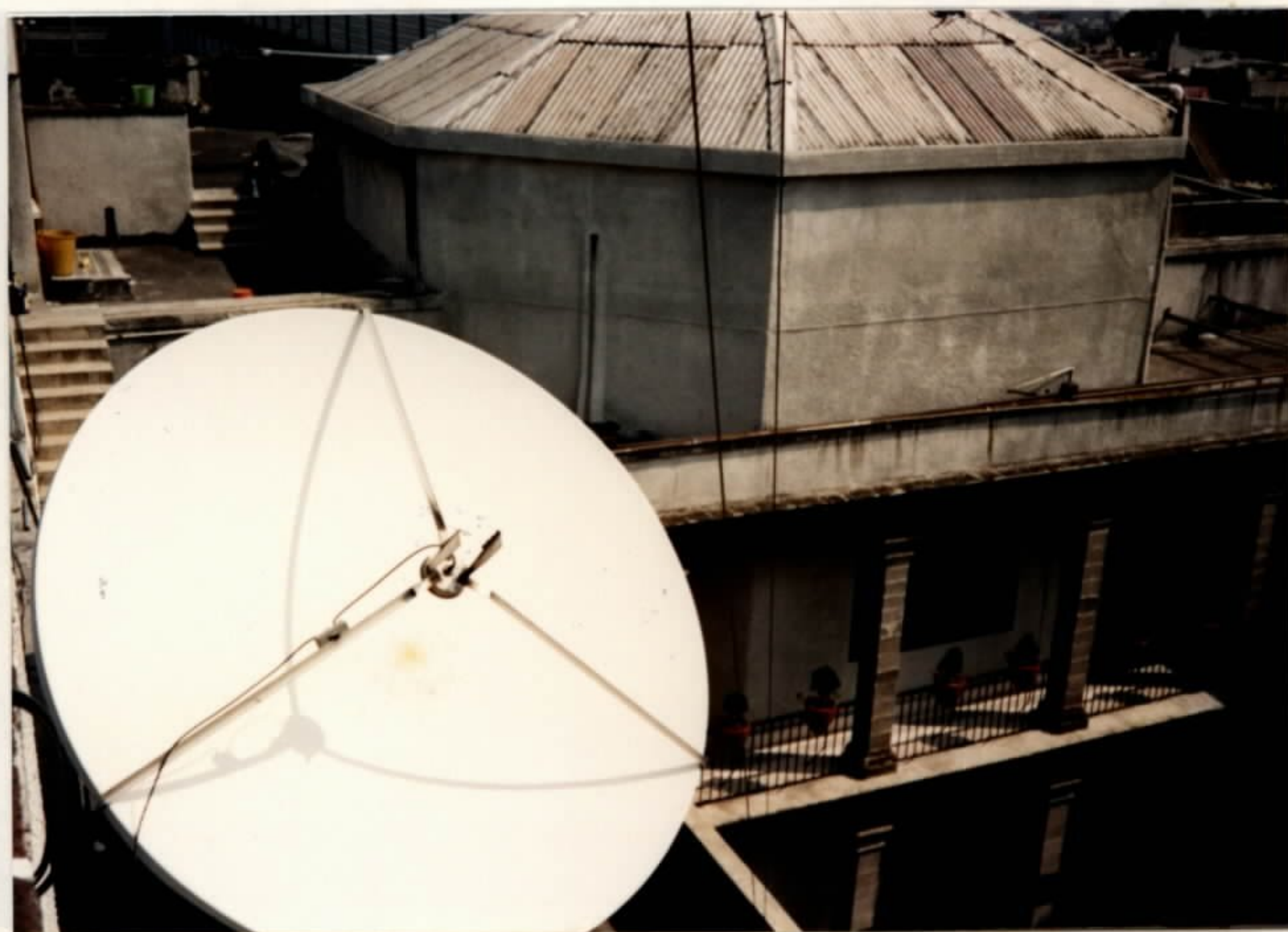
ANTENNA AT THE PENTHOUSE CNA - MEXICO
