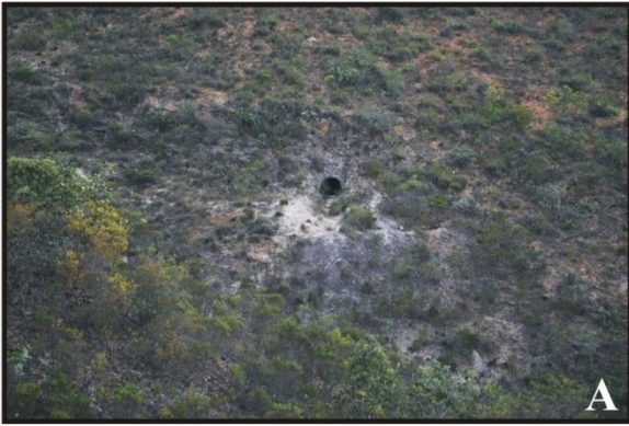
Figura 38A - Galeria antigo garimpo ás margens da BA-148, Rio de Contas, BA Figure 38A - Old gallery mining on the roadside of the BA-148, Rio de Contas, BA Foto: Violeta de Souza Martins, 2016
